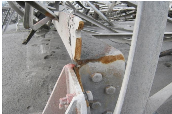
Figure 1. Failure of steel structure exposed to pyroclastic flow.
